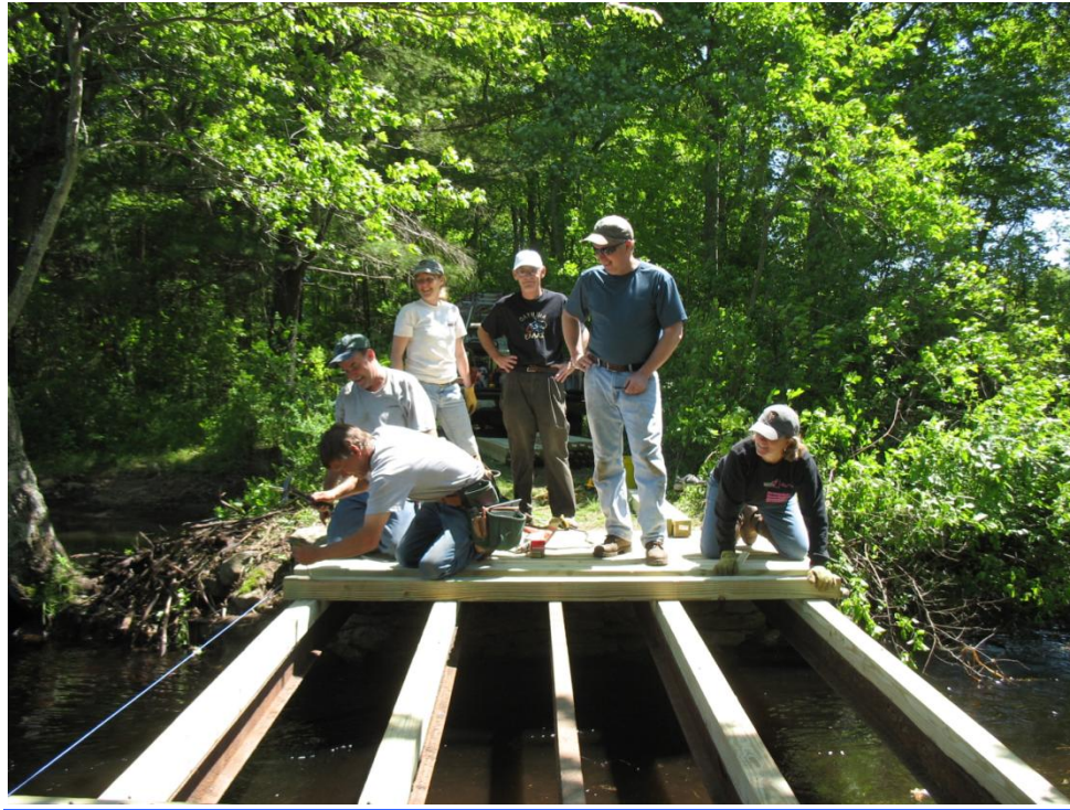
Members of the Pomfret Horse & Trail Association worked on rebuilding a bridge with a private landowner agreement they have for Hearthstone Trail in Woodstock. The PHTA had 17 volunteers come out to help that day!
